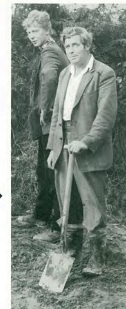
Two labourers from the Mold mains gang pause in their job of backfilling a stay hole. On the left is Mr. M. R. Jones with his companion M. V. Jones.
